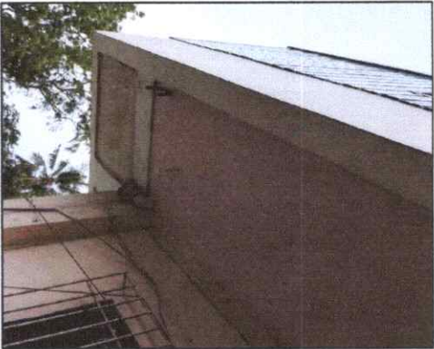
EXISTING CONCRETE CEILING AND WALL NOTE: NEED REPAINTING
